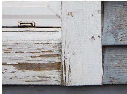
PAINTED WOOD Paint needs constant repainting.
