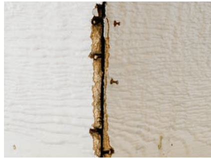
ENGINEERED WOOD Unsealed ends? Rot is coming.
