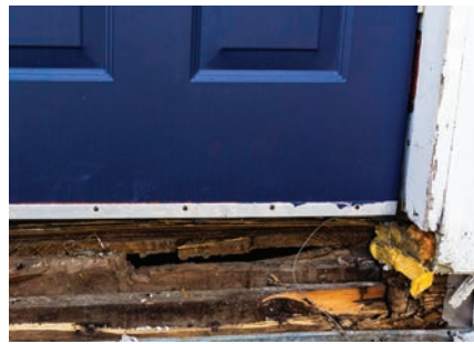
PAINTED WOOD Moisture cycles destroy wood.
